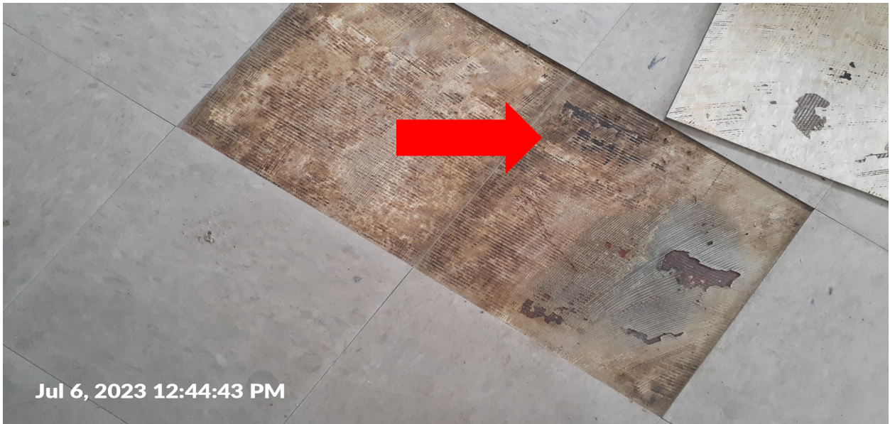
Closer view of the lobby located in Building 6 (Samples 01 and 02). The black mastic under the gray 12" x 12" vinyl floor tile was found contain 2% Chrysotile Asbestos (indicated by the red arrow).
